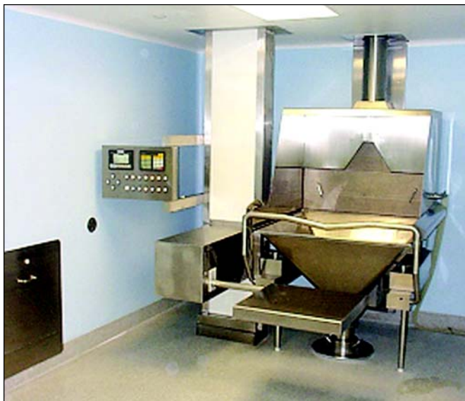
Figure 5. Weighing funnel located at the upper level.
