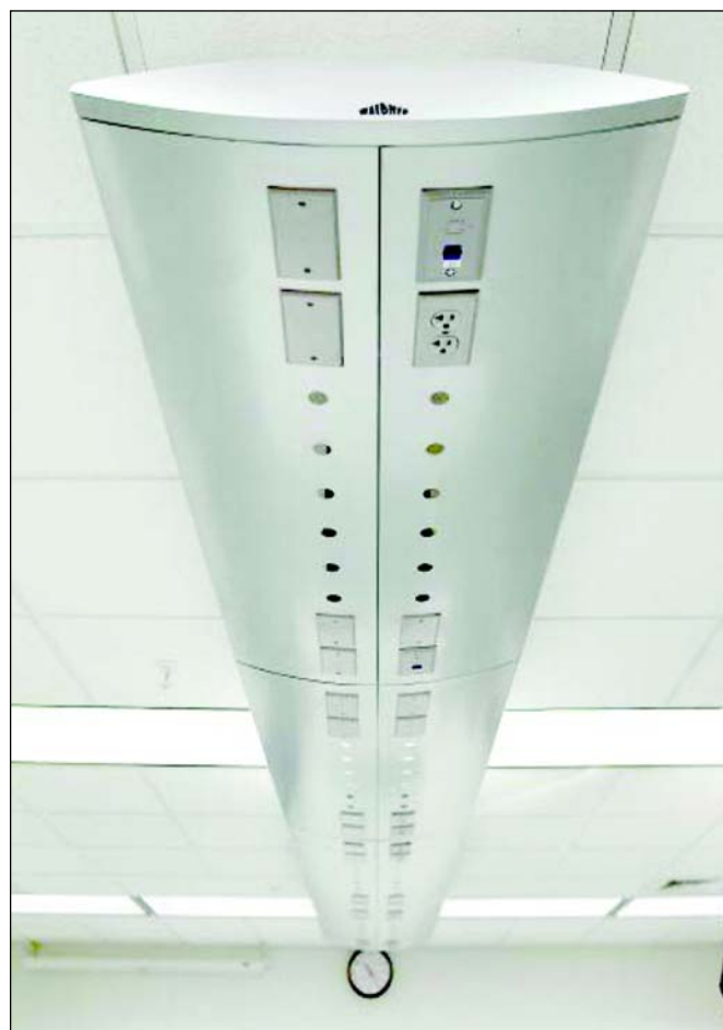
Figure 5. Overhead service carrier example. 5
