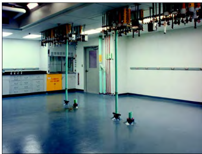
Figure 4. Utilities need to be both accessible and out of the way to promote flexibility. Ceiling mounted utilities, which are migrating from manufacturing suites to the lab, accomplish both objectives.
