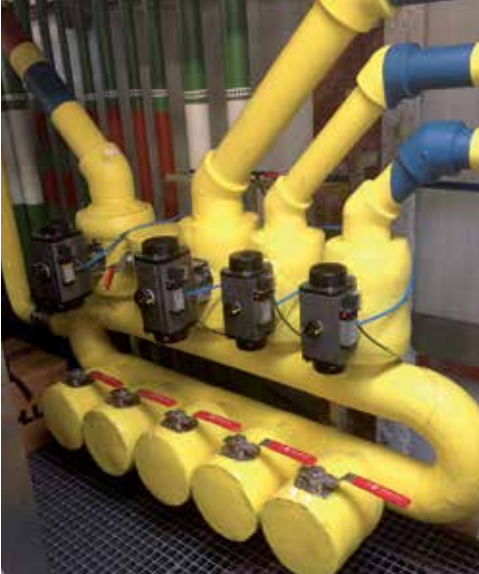
Figure 3: VPHP manifold with four outlets and spares for future use
