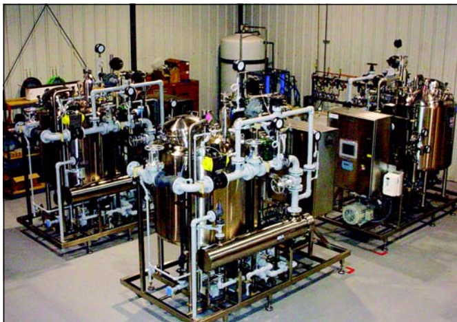
Figure 3. CIP skids configured for testing.
