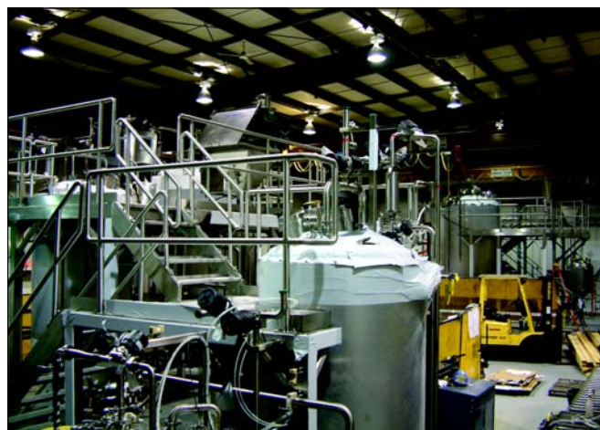
Figure 4. Buffer prep skid in supplier's facility.
