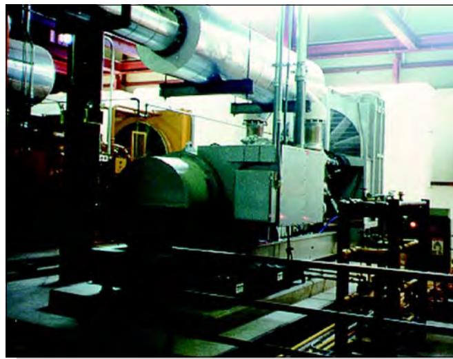
Figure 3. 1,600 Kilowatt and a 1,400 Kilowatt (background) - 13,200 Volt, 3 phase diesel engine emergency generator set.
