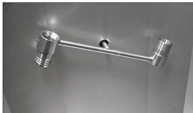
Figure 3. Ejector installation in the sterilizer ceiling.
