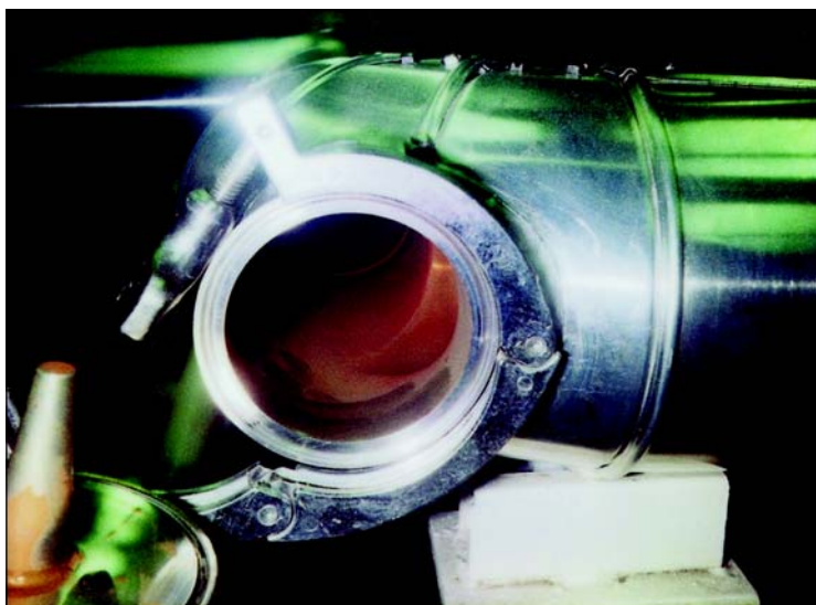
Figure 1. Rouging on the internal surfaces of a WFI system. 5
